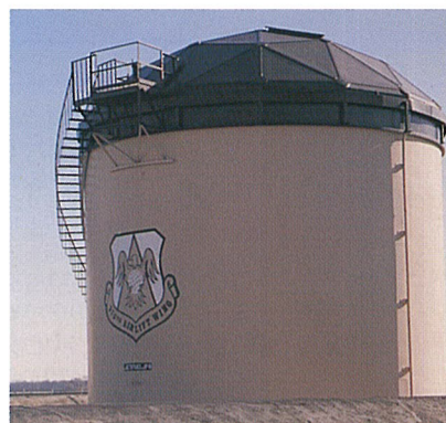
A fuel storage tank sports the base's required brown, but with the decorative logo unique to the base. EVCO stripped off the old lead-based paint, repaired the nicked and chipped tank siding, and painted the logo.
